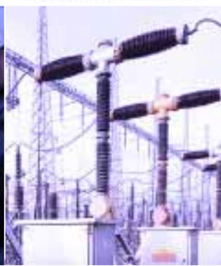
CORONA, PARTIAL DISCHARGE DETECTION
