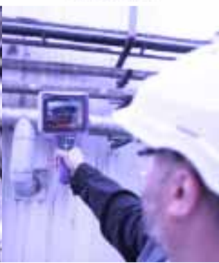
COMPRESSED AIR LEAK DETECTION
